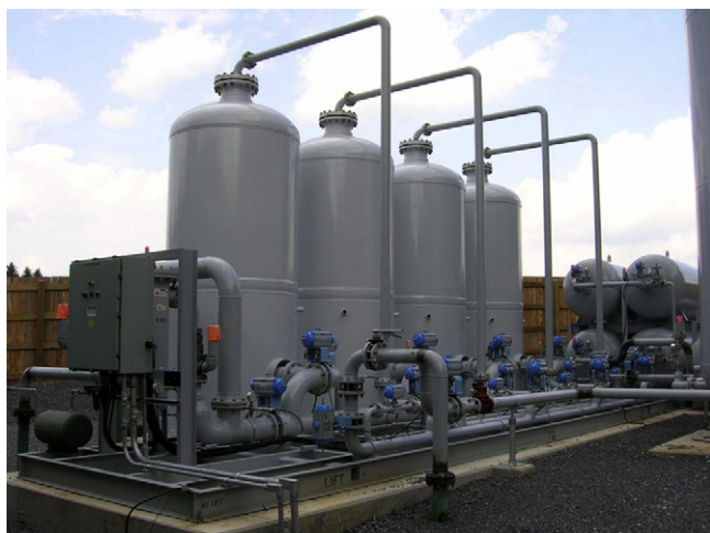
Fig. 5. Molecular Gate™ adsorption system for nitrogen and/or carbon dioxide removal (courtesy of Guild Associates, www.moleculargate.com ).
